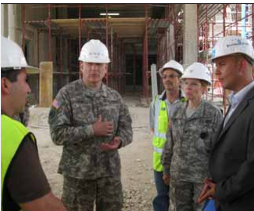
USAREUR Commander Gen. Carter F. Ham (center) visited Caserma Ederle May 26 to receive updates on the Vicenza Enhanced Health Center construction and post transformation. Construction is expected to be completed in May 2010 with a tentative opening scheduled in late September 2010. The center will consolidate health care facilities, including the dental clinic and new birthing center. Also pictured (from left): Frank Varano, Health Facility Planning Agency construction officer; Lucio Ruggiero, NAVFAC quality assurance engineer; health center commander Col. Lorraine Breen and Gordon Atkinson, contractor project manager.
